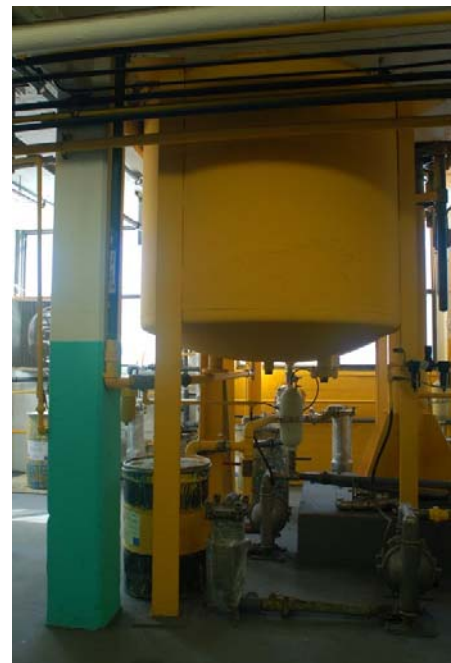
Storage vat filled by gravity flow from mixing operations on upper floor.
